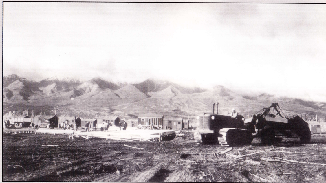
LEFT: This photo shows beginning construction of the first permanent building at the Tanacross airport. The Stout prefab houses and other buildings were used for worker housing. The truck parked at extreme left indicates that at least a winter road to Tanacross was open at this time, which Lavell Wilson estimates to be 1942. (Courtesy of Lavell Wilson)
