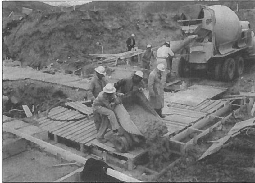
Figure 5: Construction workers pouring concrete ---Site Summit. National Archives and Records Administration. RG 77.
