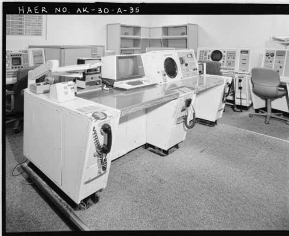
VIEW OF DATA AND ANALYSIS CONSOLE SHOWING CLOCK AND MISSILE IMPACT PREDICTOR TIME. LOCATED IN TRANSMITTER BUILDING NO. 102 AT THE CLEAR AIR FORCE STATION, BALLISTIC MISSILE EARLY WARNING SYSTEM (BMEWS), CA. 2001, LIBRARY OF CONGRESS, HISTORIC AMERICAN ENGINEERING SURVEY, HAER AK-30-A-35.
