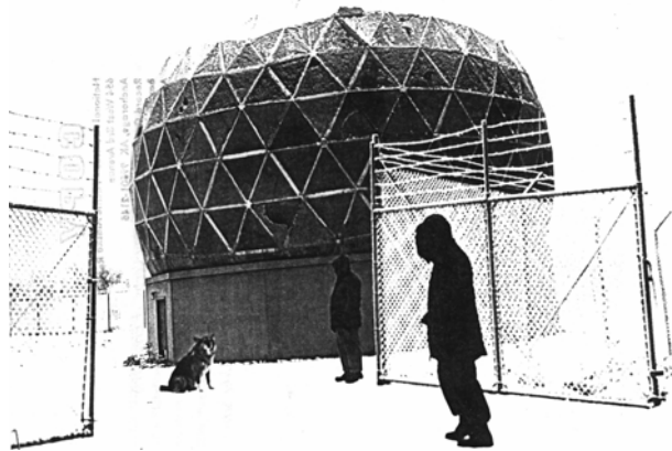
Figure 8.3 Pacific General Construction Company workmen are shown closing in the dome of a High-Power radar facility at Site Summit Nike Station near Anchorage.
