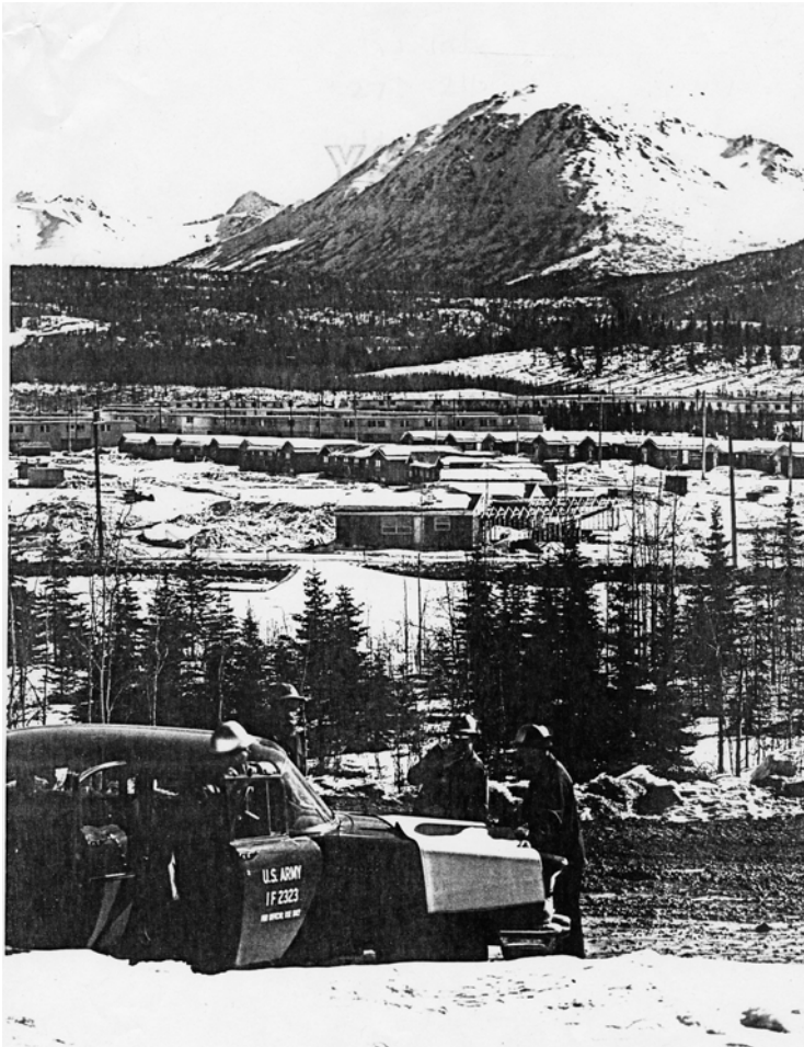
Figure 3.4 Fort Richardson Housing – Construction is well underway on 155 Army housing units at Fort Richardson, a section of which is shown in the background. Miller Brothers Company did the building under contract with the U.S. Army Engineer District, Alaska. Each unit was designed by the District for a maximum of economy and comfort. District inspectors are shown in the foreground. April 1959, U.S. Army Photo (Pending National Archives Copy, Anchorage, Alaska).
